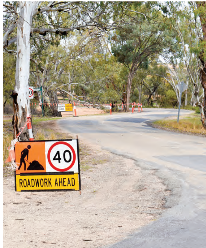
Earth works for a new river-front walking trail in Loxton along Sophie Edington Drive and Grant Schubert Drive recently began.
